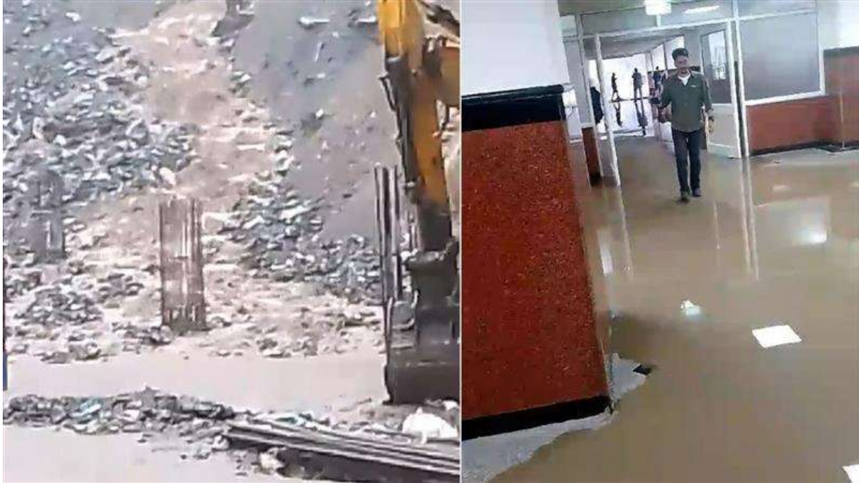
Figure 12: Water logging in new OPD block, IGMC Shimla
