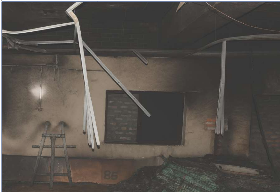
Arson / Fire Evidence
