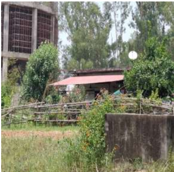
AFFECTED WIRE BOUDNRY WALL
